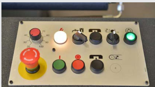
PIC: CONTROL PANEL
